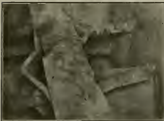
BUCKLED CENTER SILL WITH ARCHED COVER PLATE.
